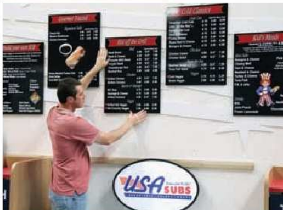
DNI Retail Design, St. Charles, Ill., has a team that can handle complete store build-outs.
